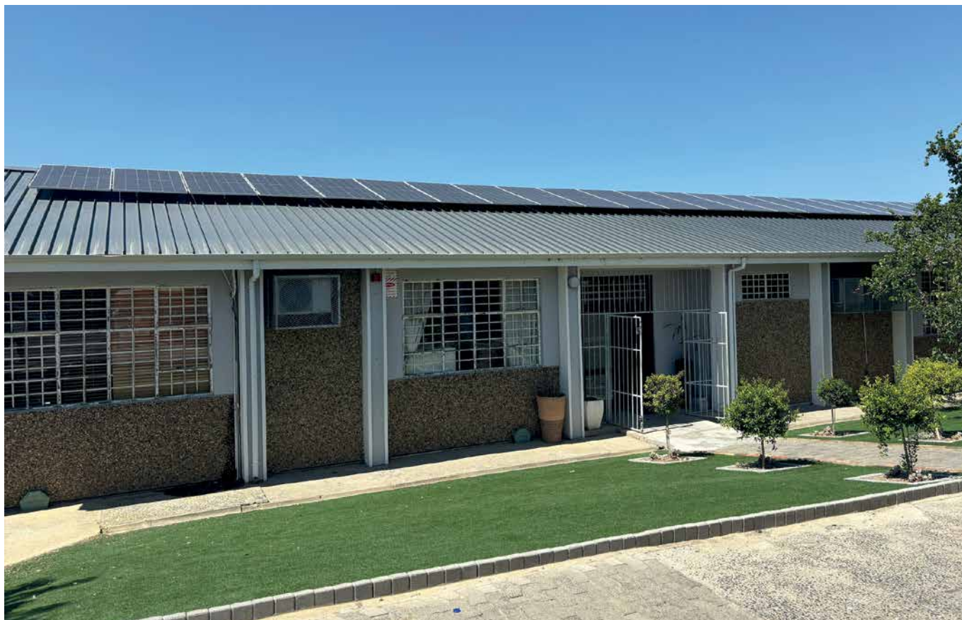
Solar PV system installed at Cloetesville High School. The hybrid inverter, panels and batteries power the whole administration block.
